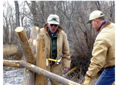
Russell Knight looks on while landowner, Ben Allen, hammers the final nail on the Hayden Creek suspended fence.
